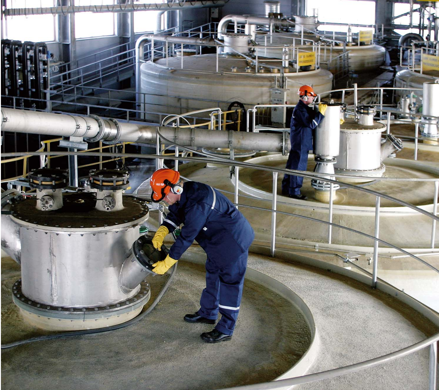
Boliden Kokkola makes use of the most up-to-date technology in its production.
